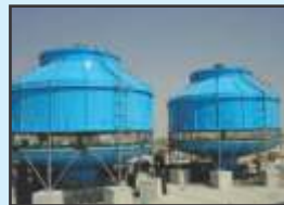
Scaling in Cooling Tower
