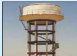
Scaling In Potable Supply Line
