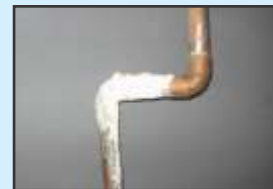
Scaling on Copper Tube
