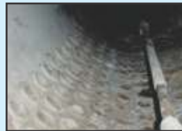
Scaling in Boilers
