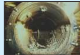
Scaling in Boilers
