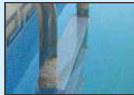
Scaling on Metal Surface
