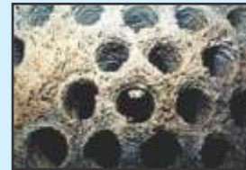
Scaling in Chillers
