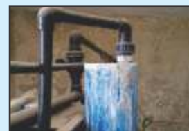
Scaling on RO Membrane
