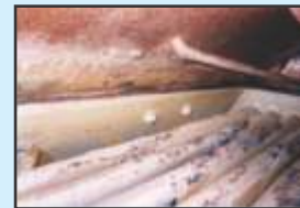
Scaling in Condenser
