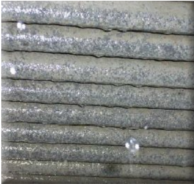
Scale thickness on tubes 75 days after installation was 0.05mm or less
