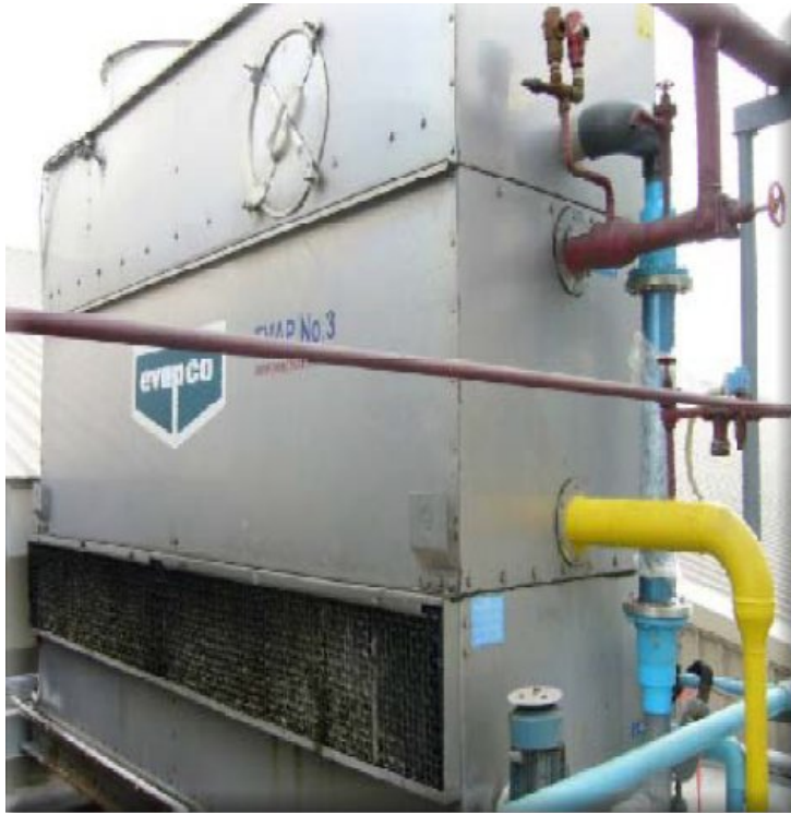
4" Colloid-A-Tron pictured on the inlet to the condenser
